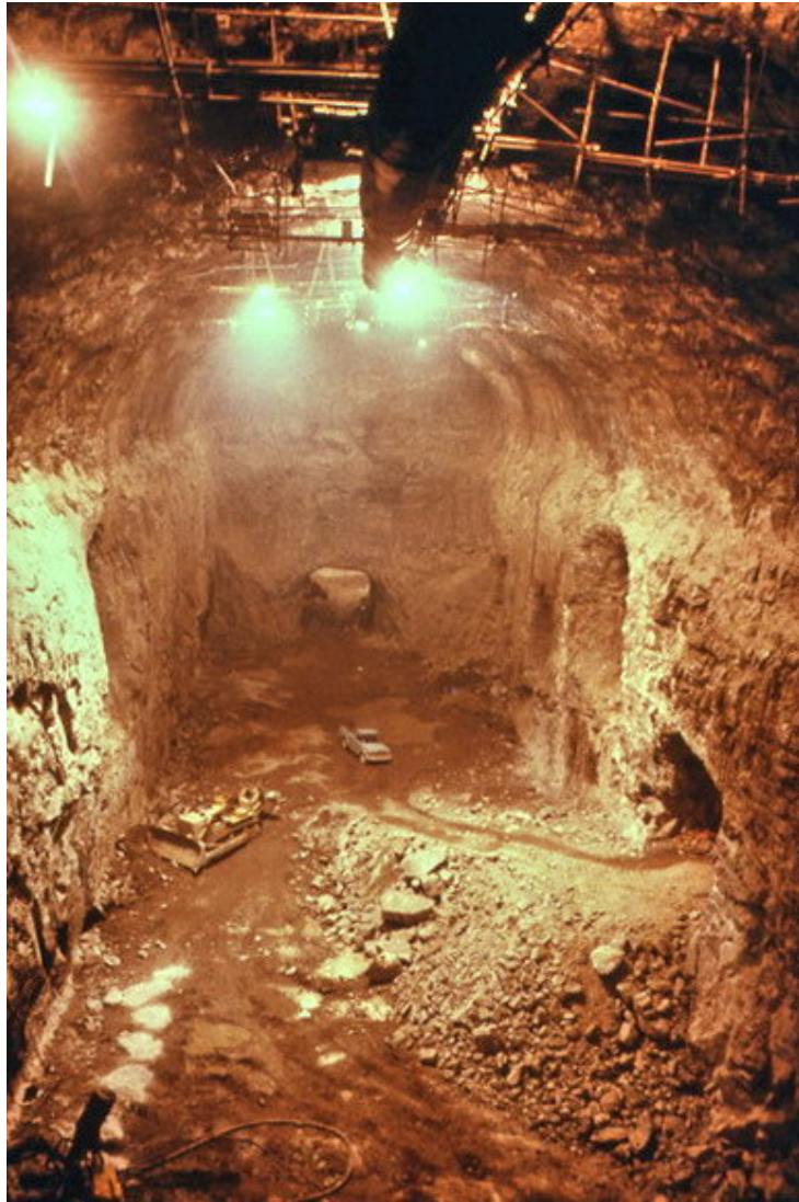
Figure 7: A view of the 25 m span Rio Grande power cavern during excavation of the lower benches.
