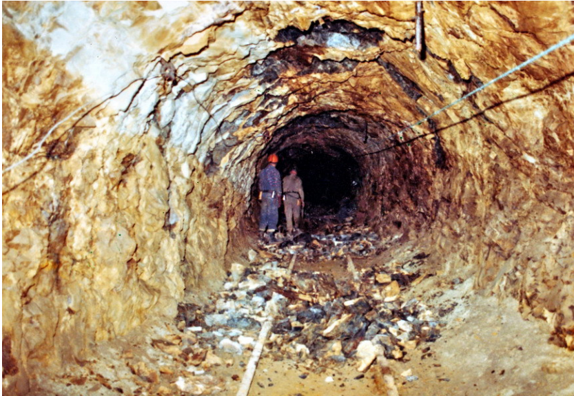
Figure 5: Ravelling of small wedges in a closely jointed rock mass. Shotcrete can provide effective support in such rock masses
